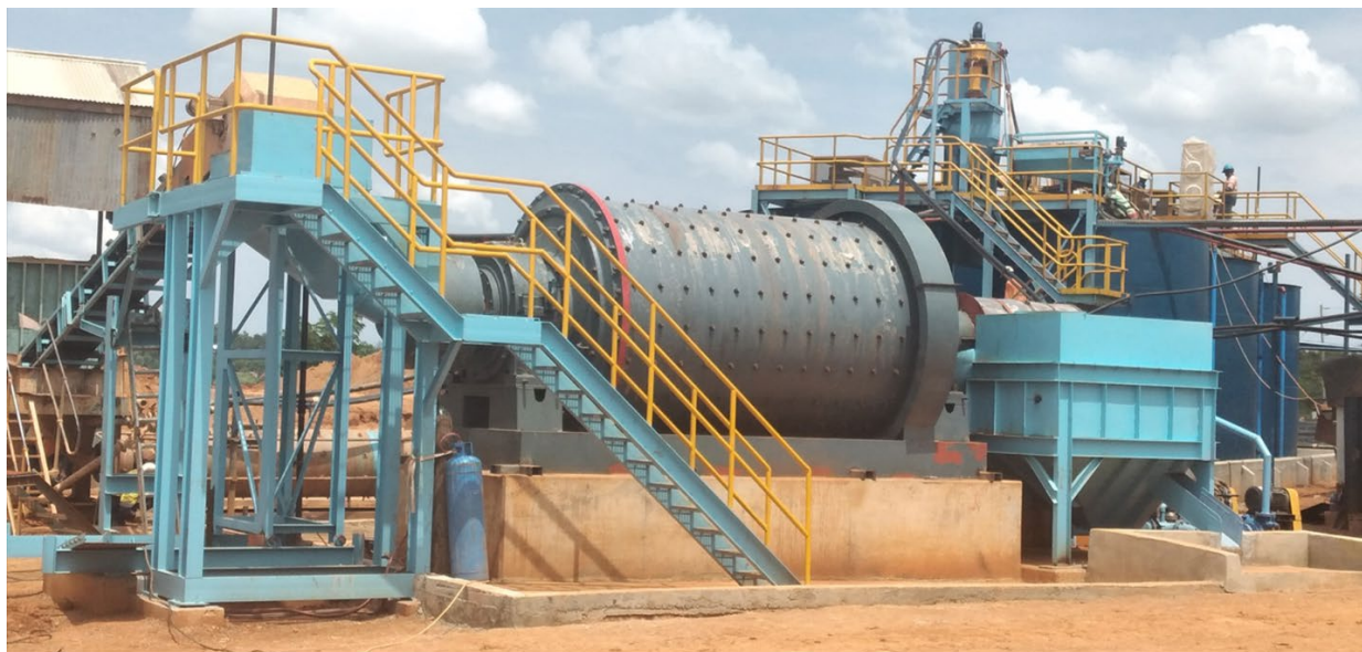
Figure 4: Buckreef Gold Expanded 360 TPD Processing Plant Integrated With 120 TPD Processing Plant (Q3 2022)
