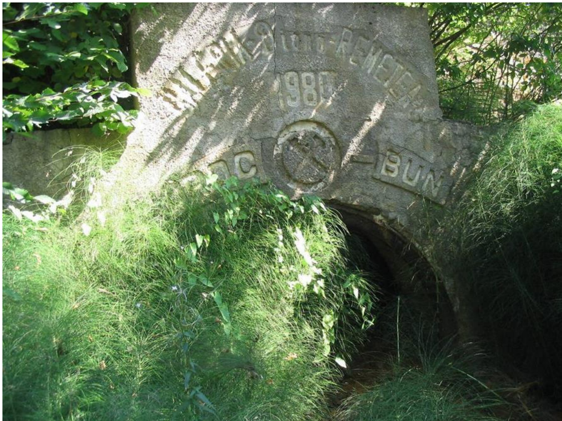
Figure 6.2: Underground Portal Now Collapsed at Rovina
