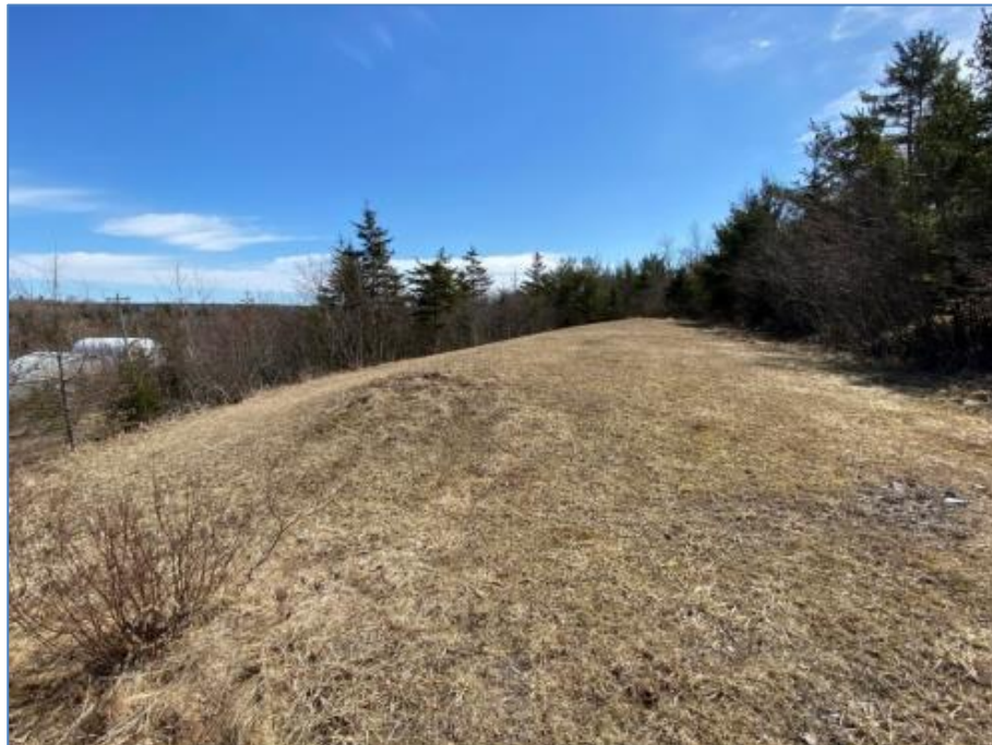
Figure 18-53: Effluent Treatment System: Septic Leach Field
