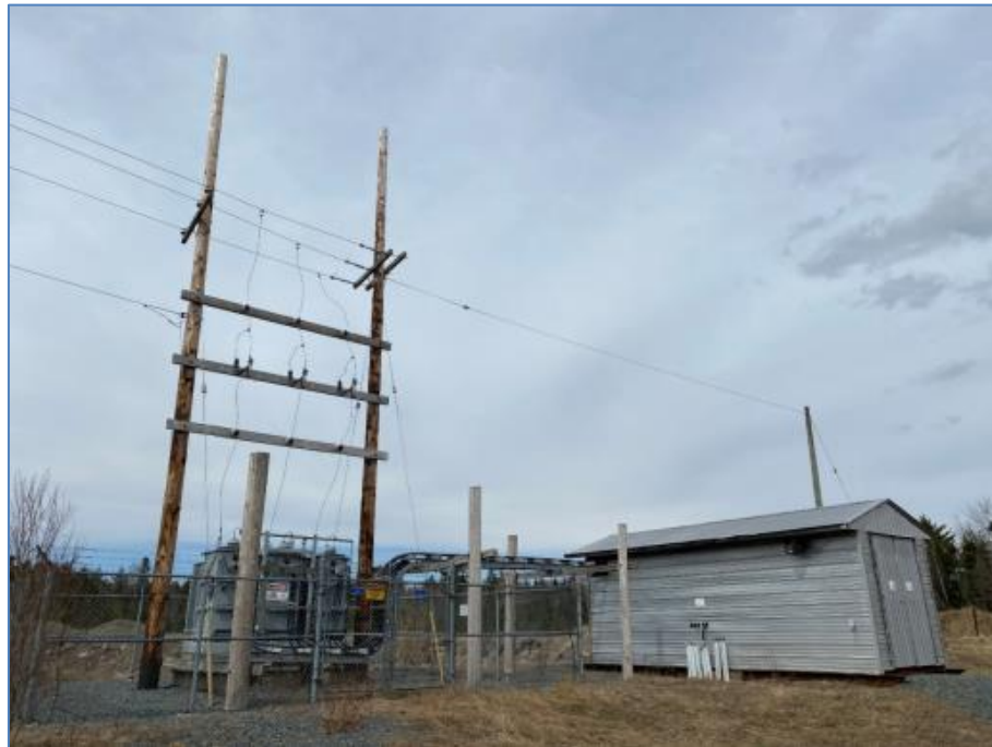
Figure 18-5: Mine Dewatering Transformer and Substation
