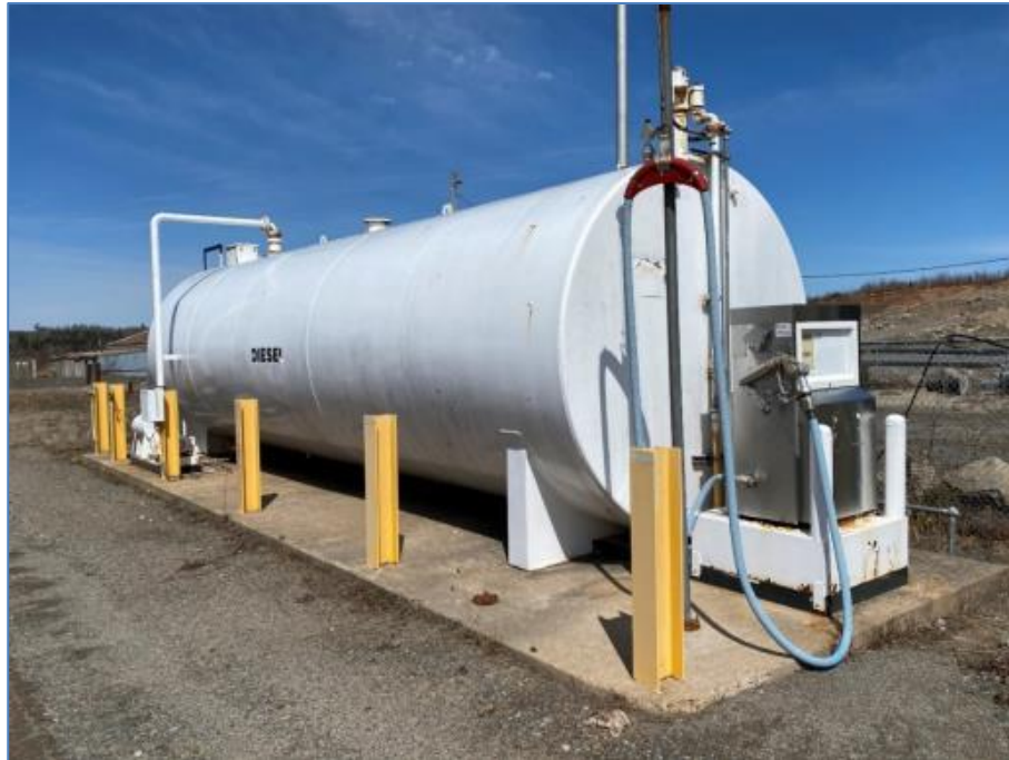
Figure 18-50: Diesel Fuel Farm
