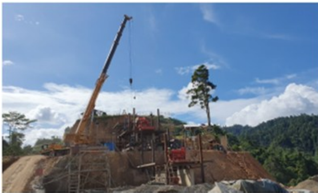
Crushing Circuit: Primary Jaw Crusher Base (CNW Group/TVI Pacific Inc.)
