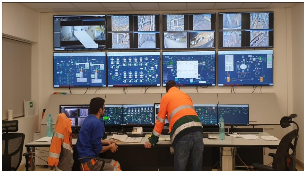
Figure 17-3: Control Room overview
