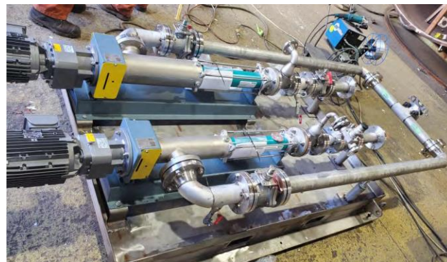
Pump skid assembly
