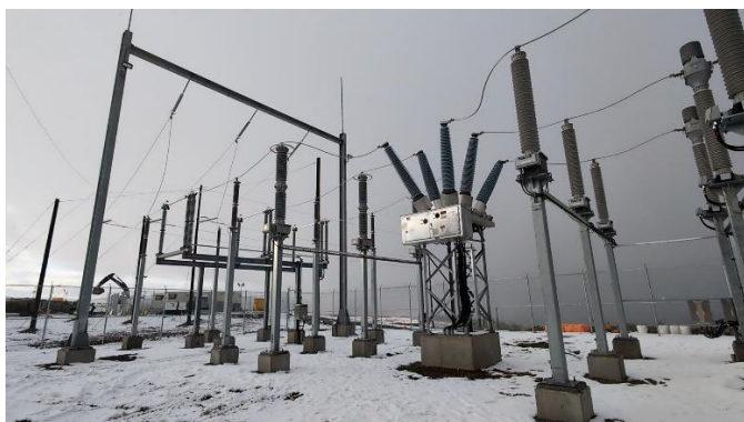
Blackwater 225kV substation
