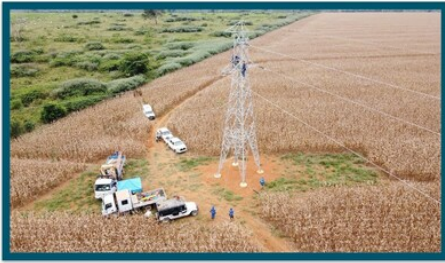
Figure 9 – Transmission Line Tower Clamping (CNW Group/G Mining Ventures Corp)
