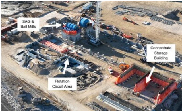
Processing Facility (CNW Group/Foran Mining Corporation)
