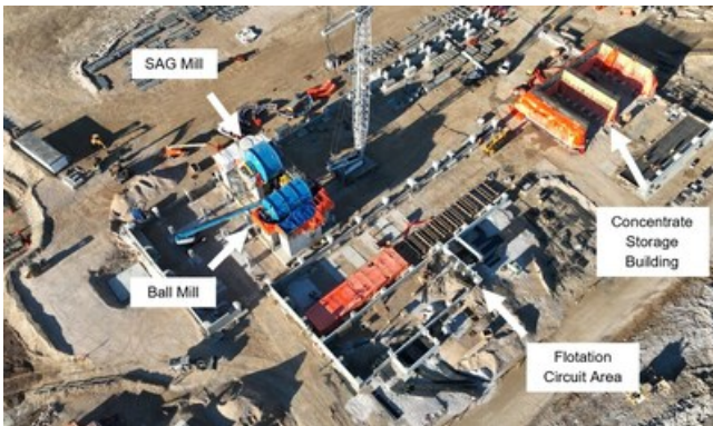
Processing Facility (CNW Group/Foran Mining Corporation)
