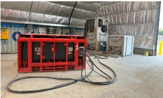
Battery Charging Station on Surface (CNW Group/Foran Mining Corporation)
